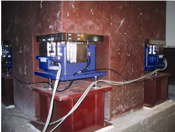
PALTCN 500 isolators located at specified points under reaction mass "C".
