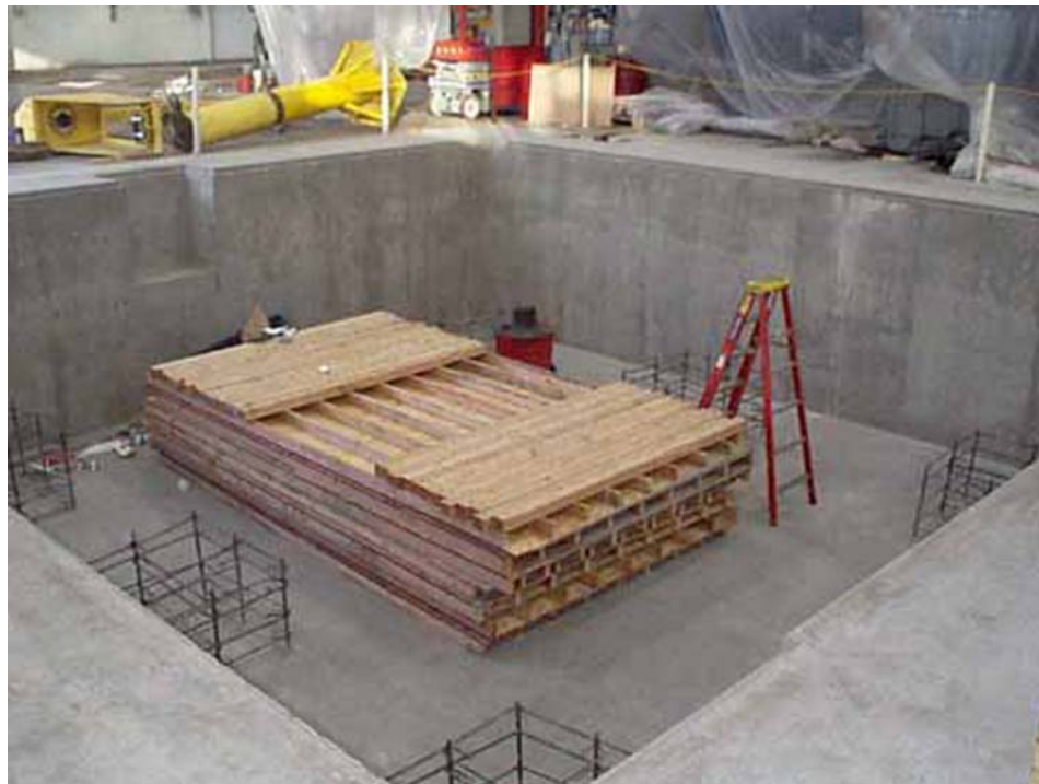
The finished pit ready for forming the mass and the isolator pedestals on the pit floor.
